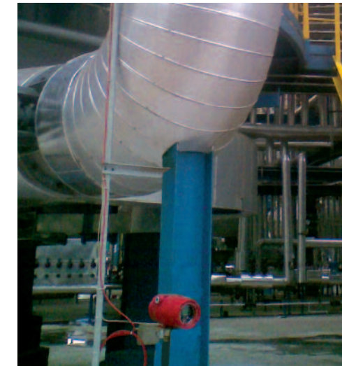
Sierra meter measuring combustion air flow in duct
